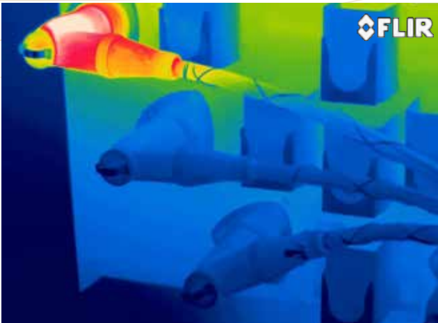
Thermal image of an overheated connection
