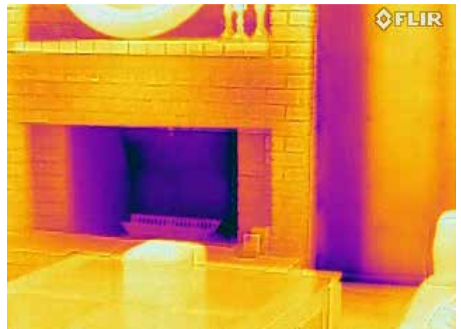
Thermal image of a fire place with MSX. Note how the individual bricks are becoming clearly visible.
